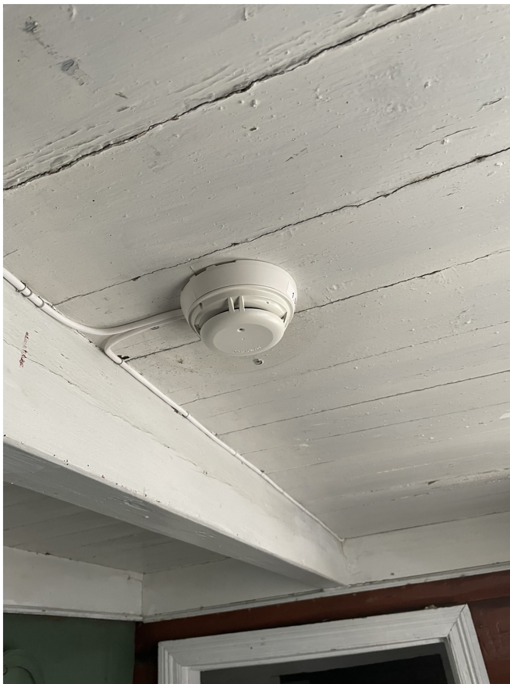
Detektorer monteret i himling.
