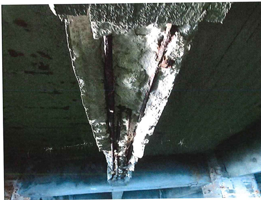
Figur 2: Brudd i bjelker under havnelager, kai C
